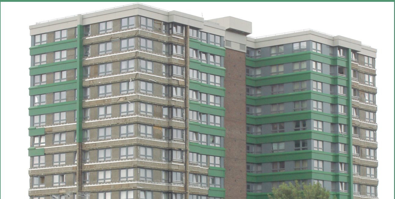
A residential tower block in Sheffield has some of its exterior panels removed with the cladding exposed for inspection following the Grenfell Tower fire, July 2017. Source: DrStrauss, Wikimedia Commons, CC BY-SA 2.0
